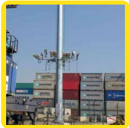
High Mast Poles
