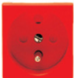
GE-OUT-1 UPS outlet
